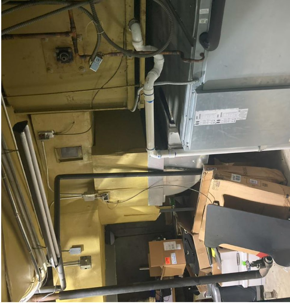
Existing Unit (Yellow) - Left Side
