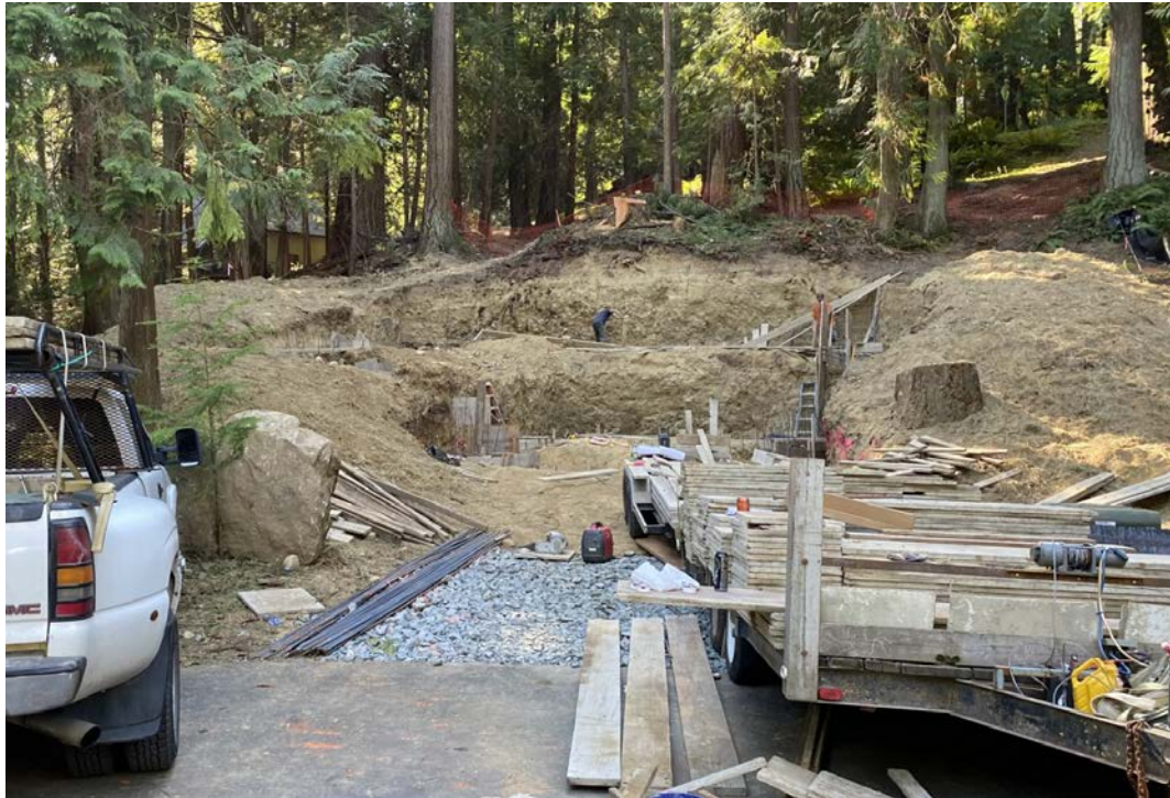
Builder errors that encroach setbacks
