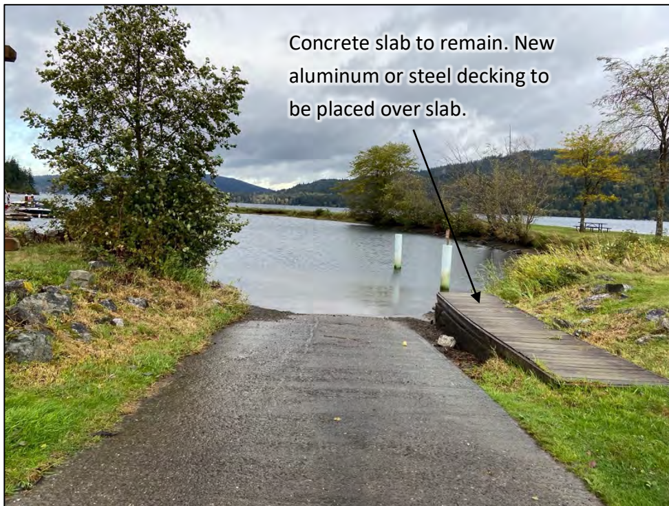
Photo 2. Existing boat ramp and concrete slab from previous dock to remain. Existing plastic-coated piles to be replaced with untreated steel piles (10/13/20).
