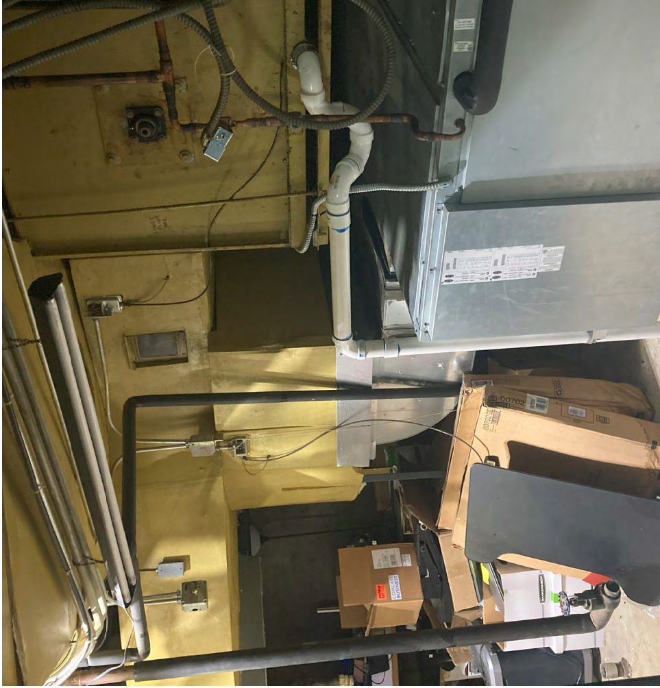
Existing Unit (Yellow) - Left Side
