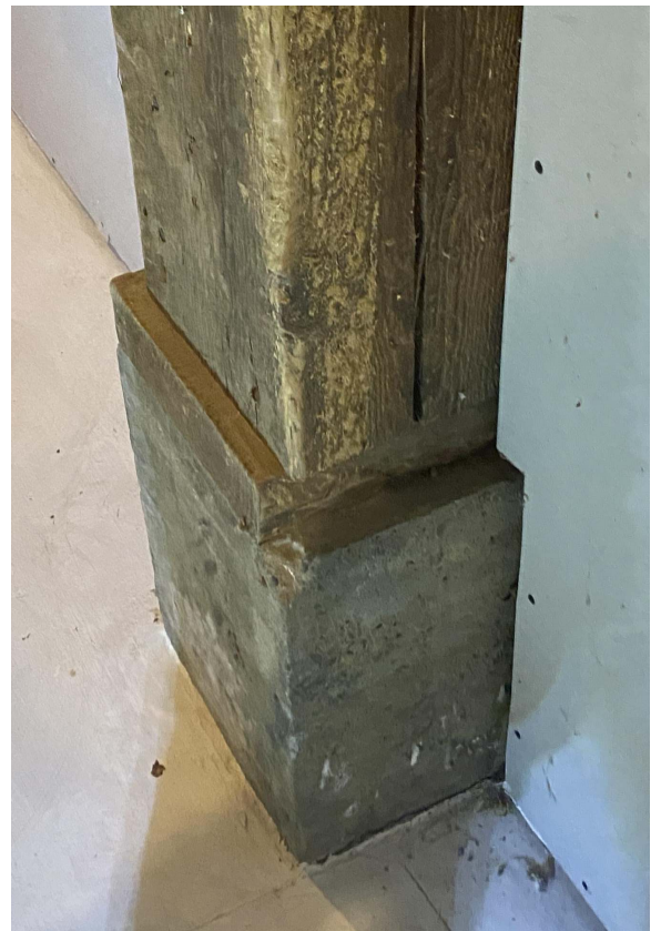
EXPOSED COLUMN IN MECHANICAL ROOM NO POSITIVE CONNECTION TO CONCRETE PLINTH
