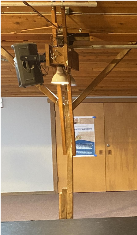
2ND FLOOR COLUMNS WITH VISIBLE LEAN
