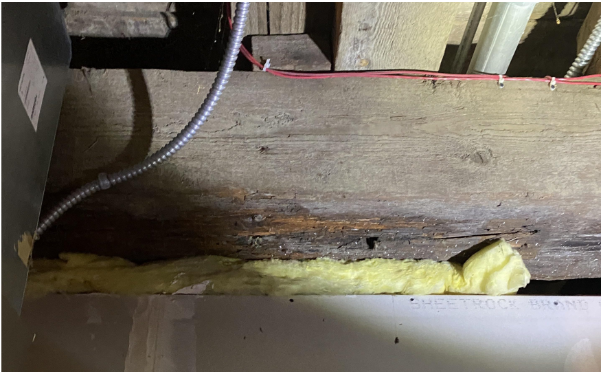
EXPOSED VISIBLE DRY ROT AT BEAM IN MECHANICAL ROOM
