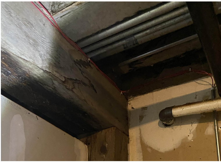
EXPOSED BEAM IN MECHANICAL ROOM WITH WATER STAINS AND NO POSITIVE CONECTION AT BEAM TO COLUMN
