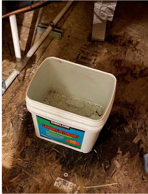
ATTIC WATER FILLED BUCKET OVERFLOWING
